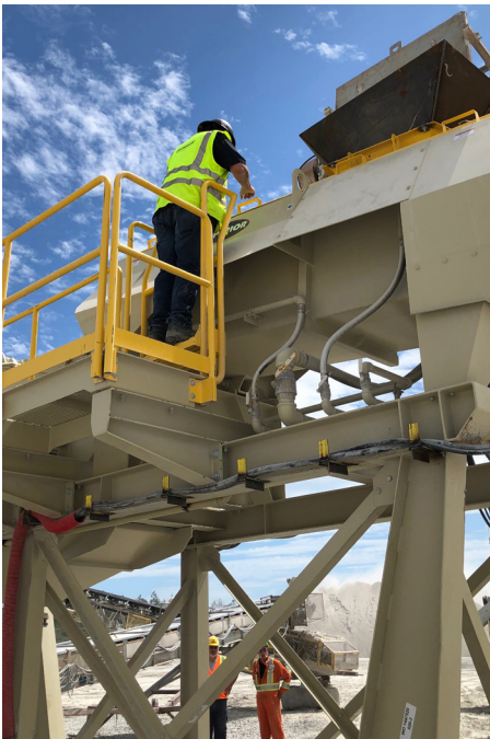
WET SCREW MAINTENANCE
